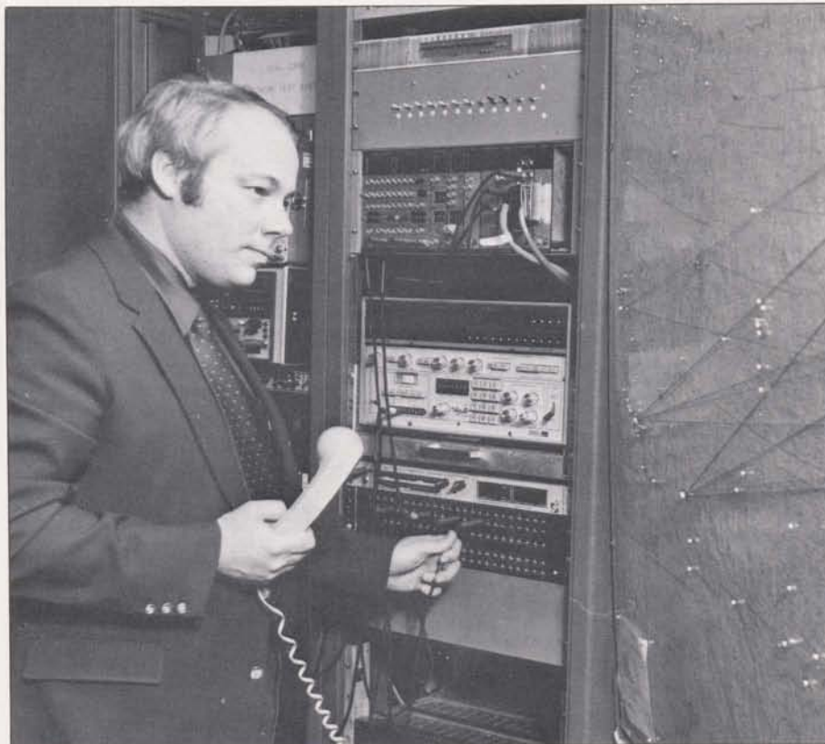
Steve Scott, manager, voice network operations and project leader of the recent cutover of DIAL-Comm, checks out the system's status.
